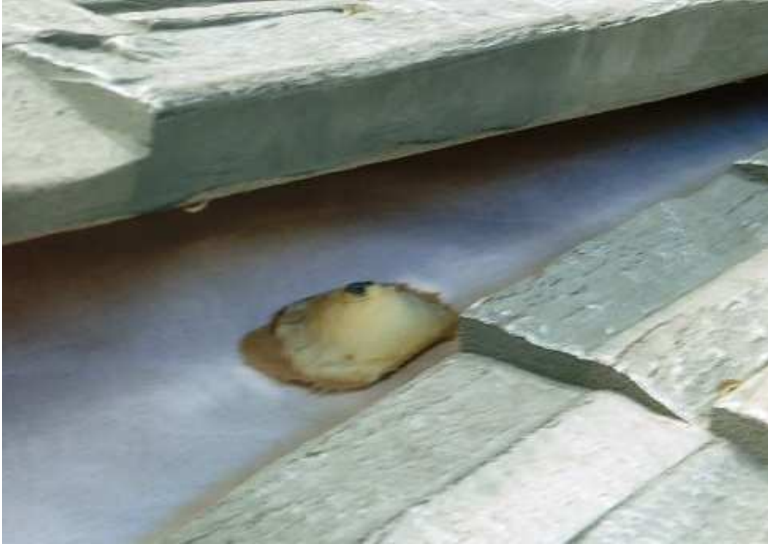
Photograph No.3 Typical results of the negative load test Fasteners pulled through the foam panels
